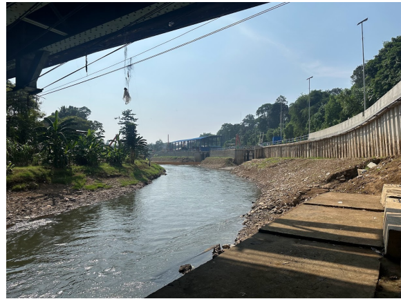
Evidence of Normalisasi through the construction of floodwalls along river (on the right)
